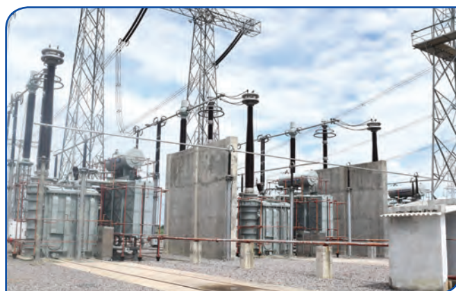
765 kV Anpara-Unnao S/C Transmission Line from Anpara to Unnao at Uttar Pradesh, financed by REC.
